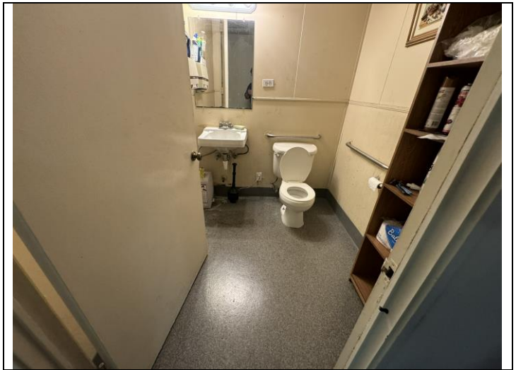
20. View of Gray Linoleum/Mastic with >1% asbestos in 178 South 6 th Avenue restrooms.
