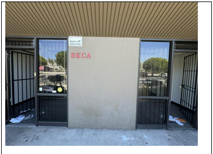
24. View of typical brown paint on exterior ceramic entry wall with lead >1.0 mg/cm 2 .
