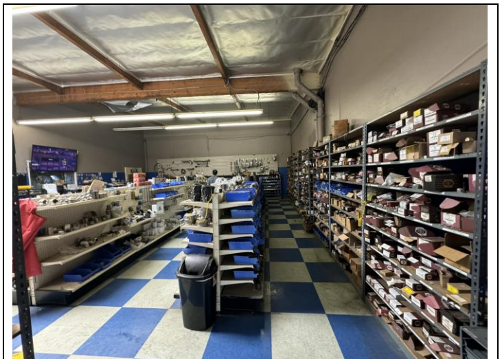
18. View of White 12"x12" VFT/Mastic with >1% asbestos in 184 South 6th Avenue store, offices and restrooms.
