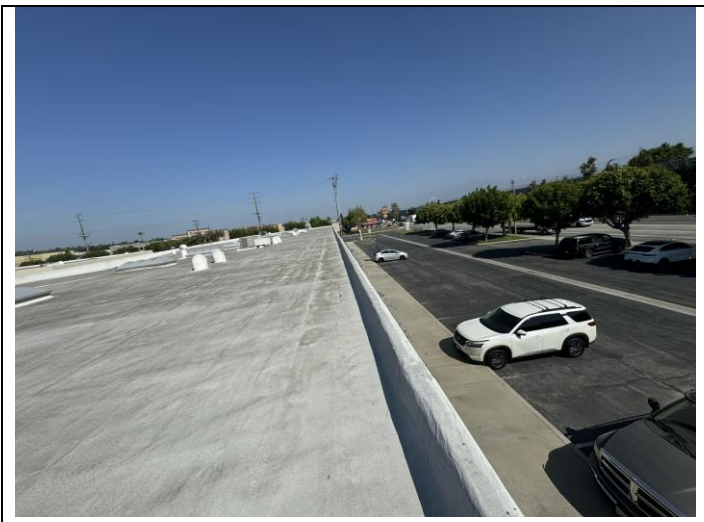
17. View of typical parapet wall cap seam mastic with >1% asbestos.
