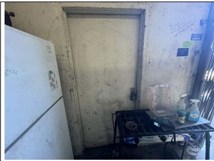
23. View of Cream Paint on metal door frame with Lead >1.0 mg/cm 2 at 184 South 6 th Avenue warehouse door.
