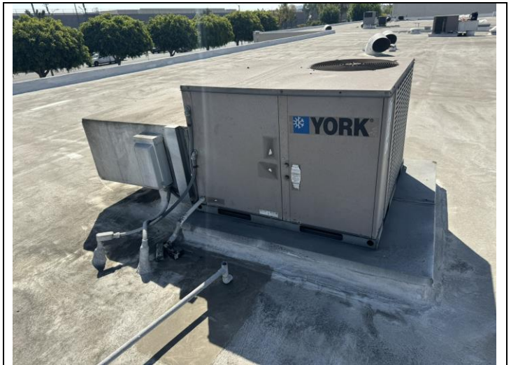
16. View of typical roof penetration mastic >1% asbestos at base of roof HVAC units.
