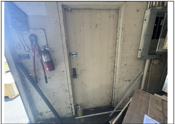
22. View of Cream Paint on metal door and door frame with Lead >1.0 mg/cm 2 at 190 South 6 th Avenue warehouse door.
