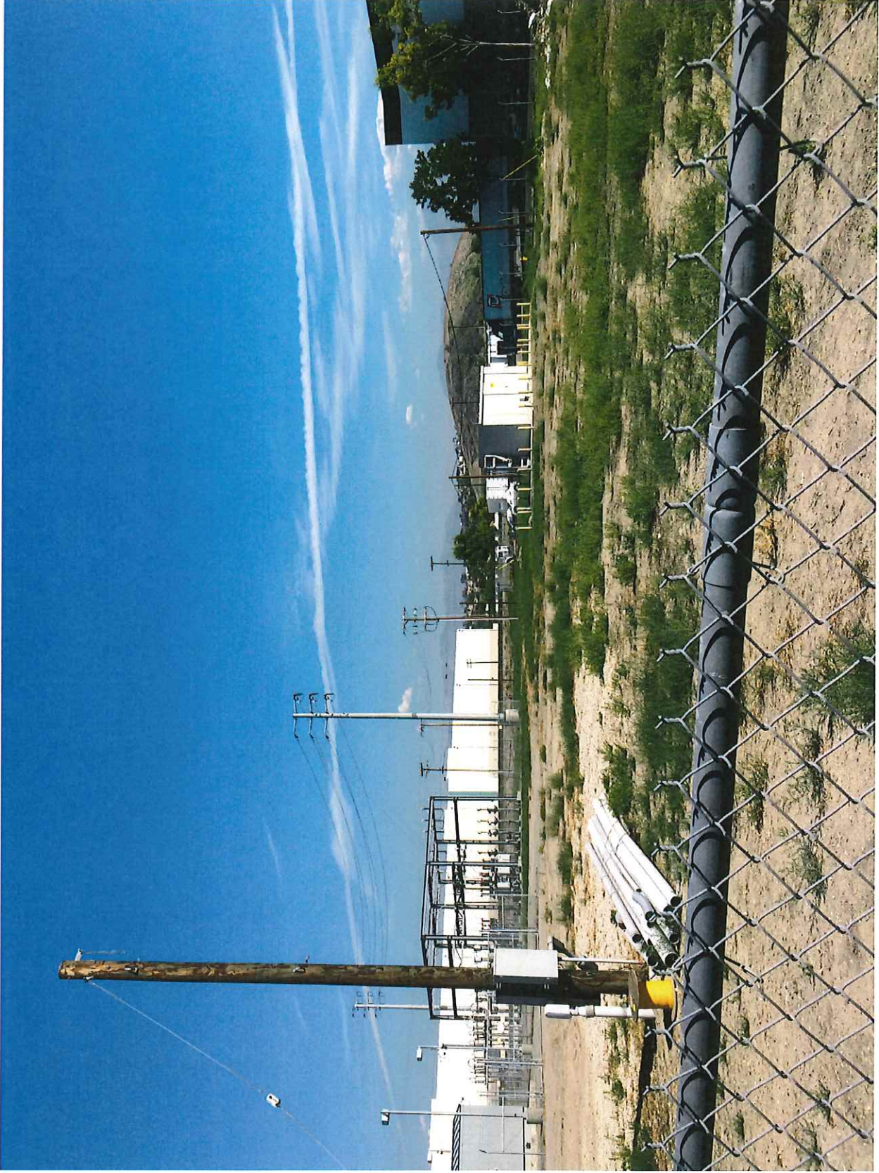
WADDINGHAM 12KV INTERCONNECTION
