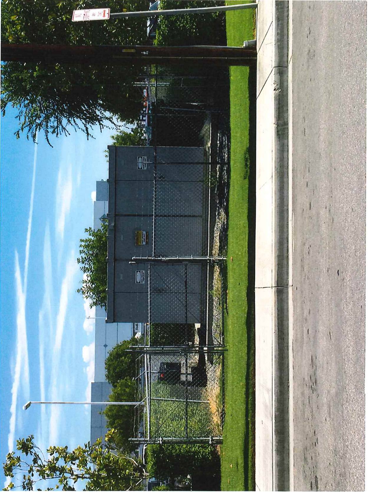
LIBBEY 12KV INTERCONNECTION
